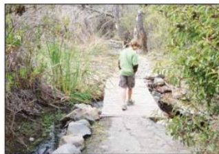
Drainage requiring improved bridge crossing or trail reroute as part of the San Diego River Trail improvements (MG-R2)
